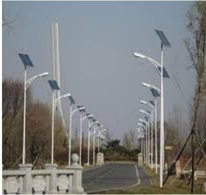
STREET LIGHTENING IN THE STATE
