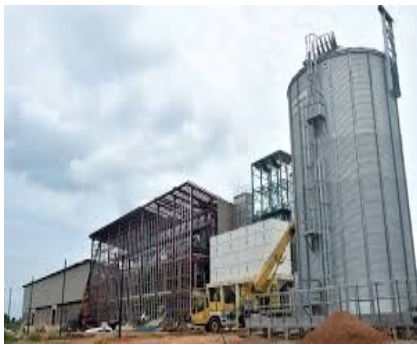
Figure 3 COCOA PROCESSING PLANT
