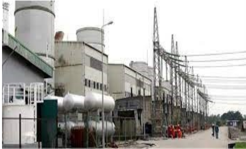
Figure 1 CRS POWER PLANT
